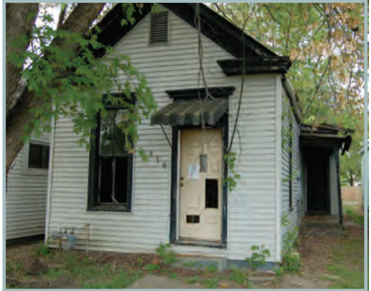
New Directions acquired this shotgun house with NSP funds. Due to extensive deterioration it was demolished and is being rebuilt using a similar footprint.
