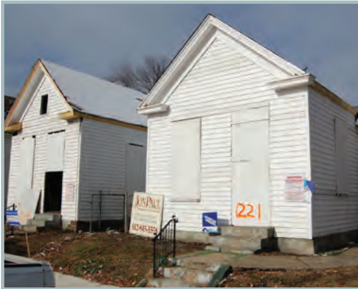
Two houses on Culbertson that New Directions acquired and is renovating with NSP funds. New Directions is adding a one-room addition to the one on the left to enlarge it and improve its marketability.
