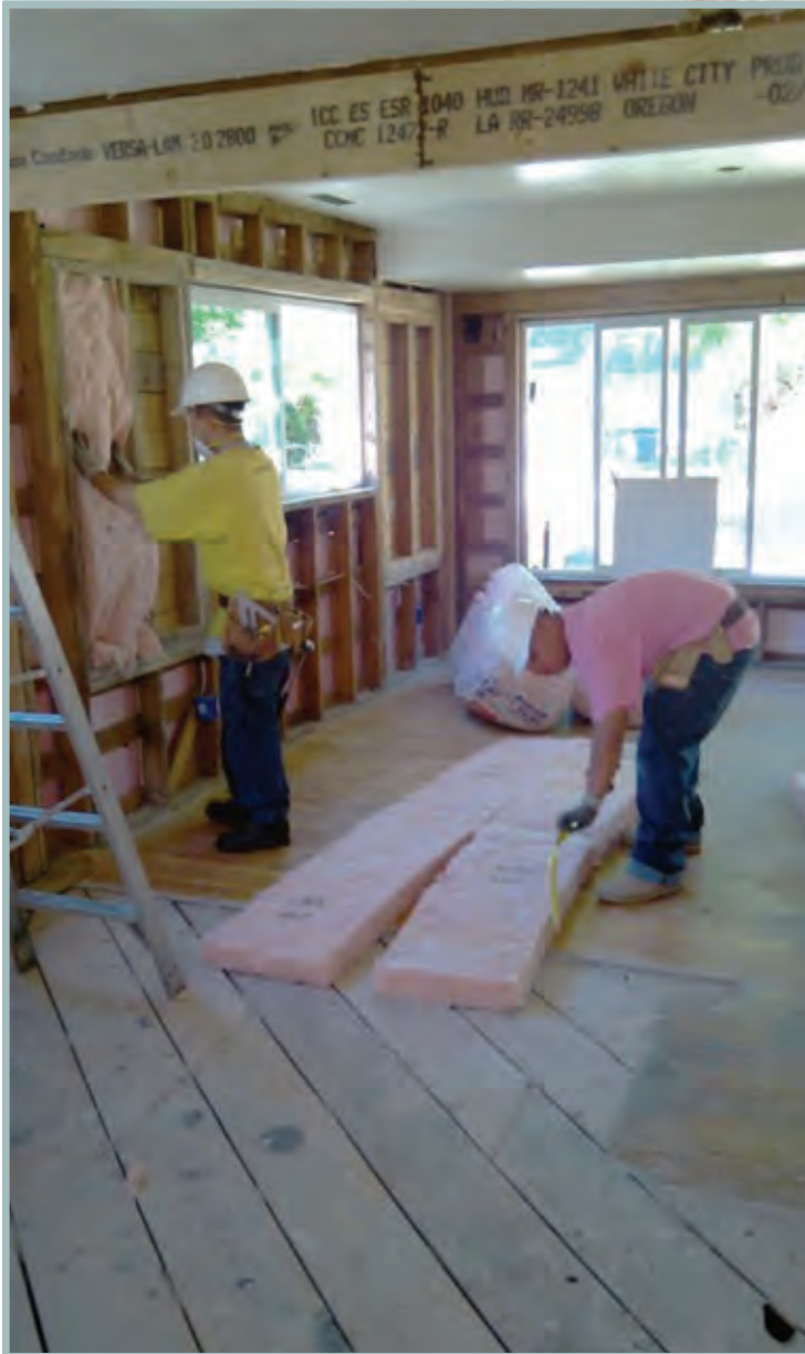
Two members of NWSL’s YouthWorks crew remodeling the first UCAH home. Among other improvements, the crew added a third bedroom and a new garage.
