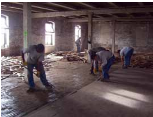
Workers for The ReUse Center engage in salvage operation while deconstructing a building. Photo courtesy of The ReUse Center
