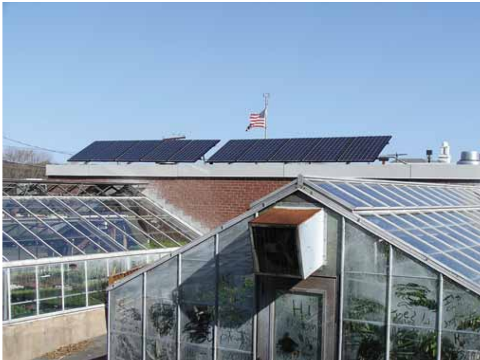
PV Squared installation at Middletown, CT Public School. Photo courtesy of PV Squared
