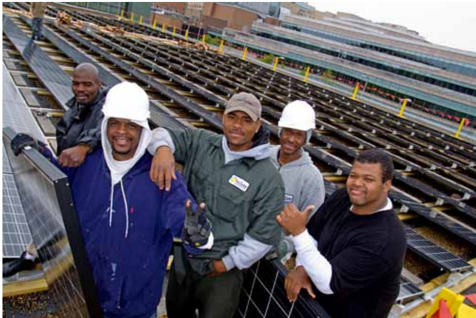
Ohio Cooperative Solar's work crew completes the first 110kW solar installation on the roof of a Cleveland Clinic building. The co-op plans to install 3MW of solar in Cleveland by 2013. Photo courtesy of The Cleveland Foundation
